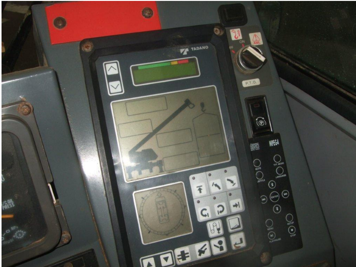
Equipment: Tadano GR 300 EX (9184) LOCATION: Belgium
